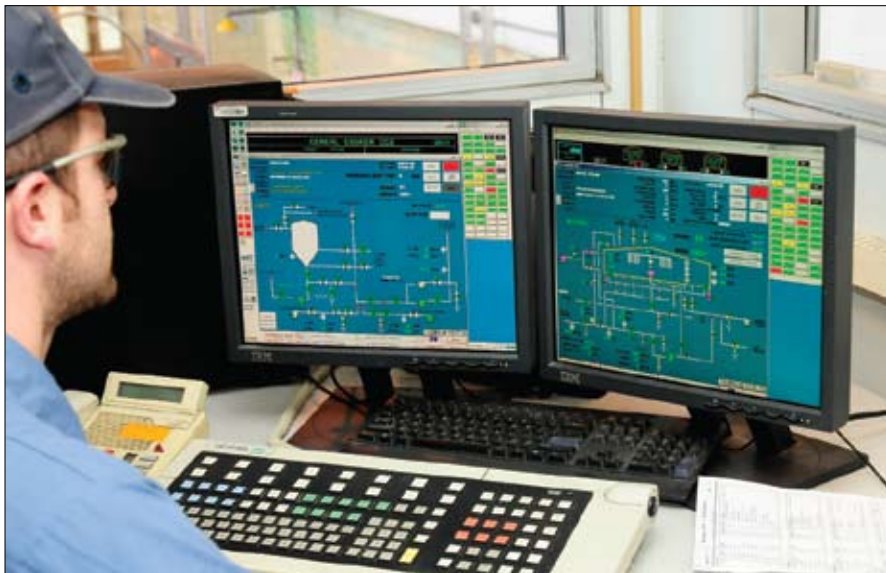
Left: Brewhouse control panels are used to monitor the processes and control product flow.
